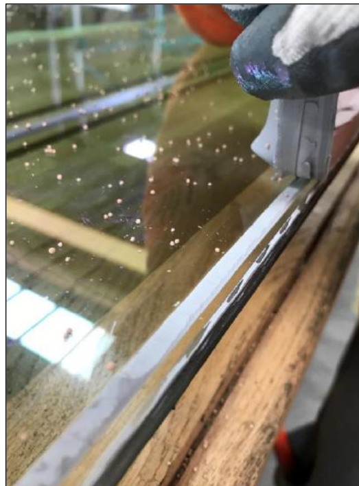
Figure 36: Adhesive failure, deglazing test negative
